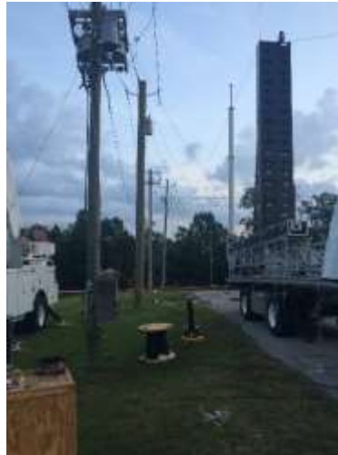
All Poles and Test Leads
